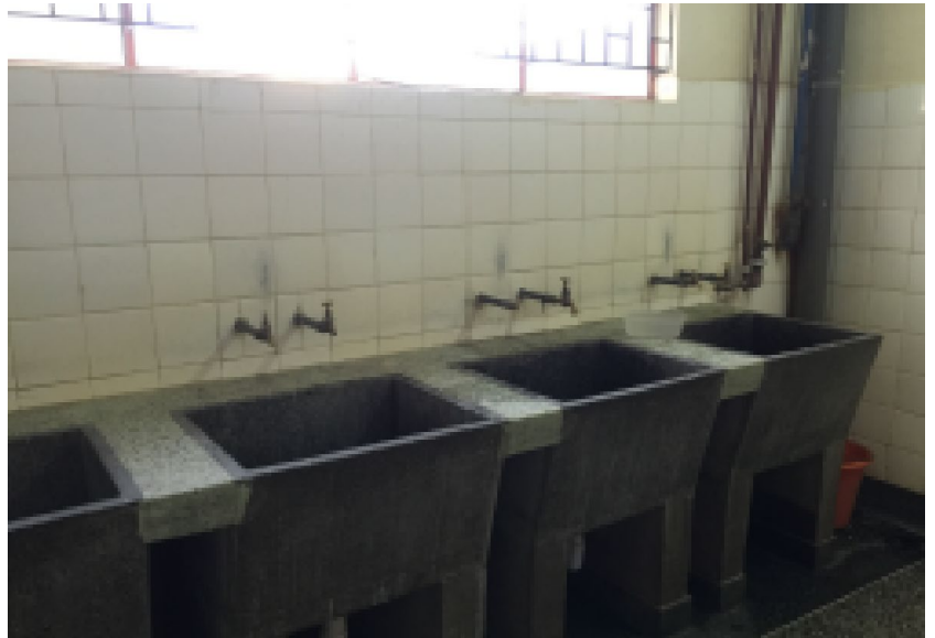
Laundry/dish washing room
